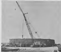
New debalasting Tank 402 will be six times the capacity of the present tank of 30,000 barrels.
